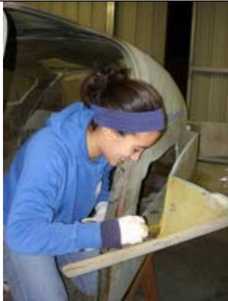
Anjuli Nunn, 1/3 of the Velocity construction team, glasses the port side strake.
